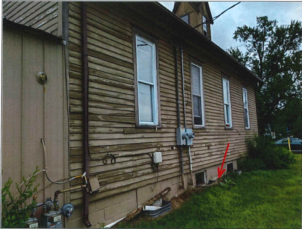
Photograph 9 - View of the west side of the church facing south and basement exterior waterproofing (Sample11a)
