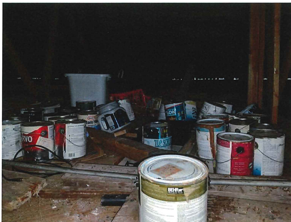
Photograph 35 - Paint containers in the garage attic.
