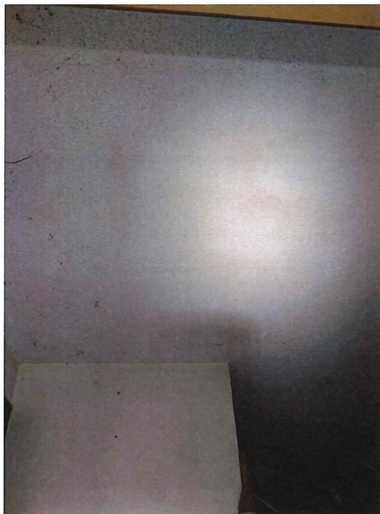
Photograph 28 - View of the ceiling in the show room area in the garage.
