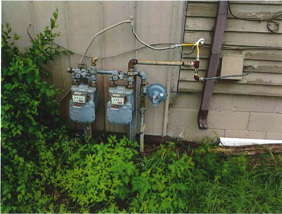
Photograph 33 - Natural gas meters.
