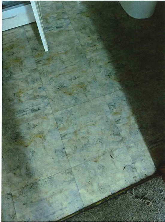
Photograph 29 - View of the bathroom floor tile in the garage showroom.
