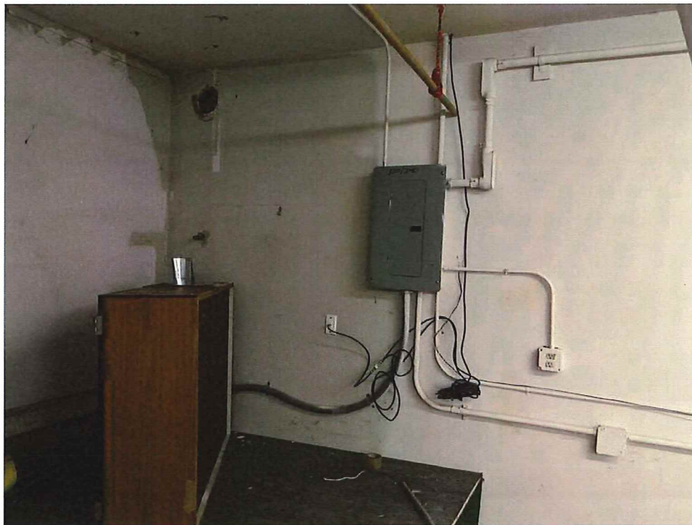
Photograph 24 - View of the electrical panel.
