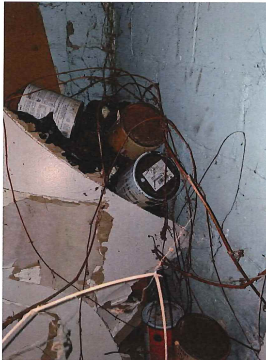
Photograph 60 - View of the paint cans behind the bedroom wall in the basement.
