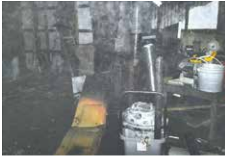
Woodburning stove not properly maintained.
